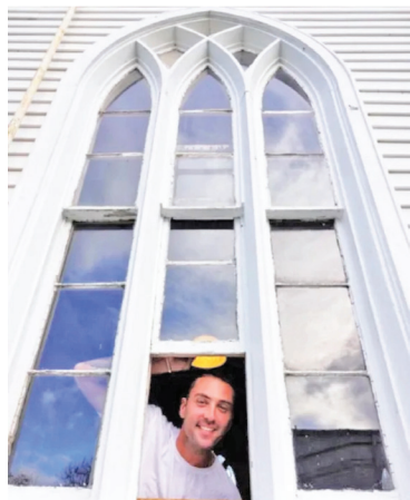
An employee of Renuitt Builders peers out the window that now opens.
